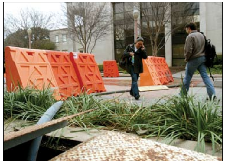
Students weave through barricades, water and hoses Monday between the Hankamer School of Business and the Speight Plaza Parking Garage after a broken water line left the area damp Sunday evening.
