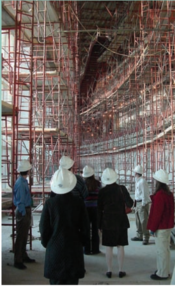
Construction officials lead a tour of the four-story glass atrium in the nearly completed Baylor Sciences Building. The building will be ready for students in the fall.
